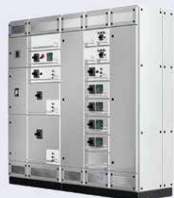
CCM Power Centre
