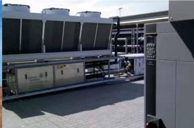
Two VLT® Advanced Active Filters for HVAC installed at a hospital to ensure a stable supply for vital equipment.
