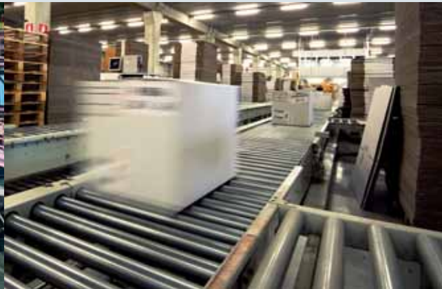
Six cost optimized VLT® 12-pulse drives incl. transformer installed at facility for material handling.
