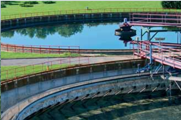
Three VLT® Low Harmonic Drives installed at waste water station ensure compliance with IEEE519.
